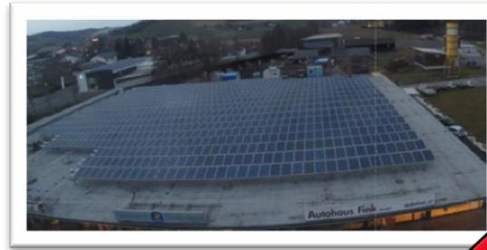
200 KWp in Gnas/Stmk
